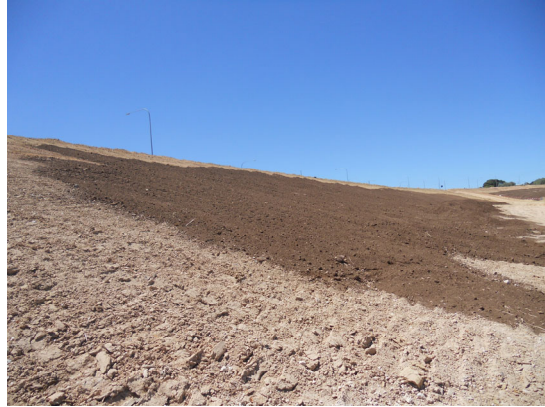
Batter subsoil has been deep ripped horizontally across the batter allowing moisture infiltration and minimising erosion potential.
