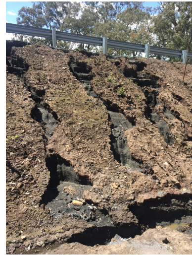
Severe erosion caused by steep batter gradient, poor subgrade material, and lack of soil preparation.
