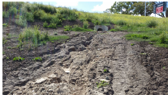
Drainage outlet located above toe of batter causing erosion.
