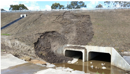
Land slip from overland flow above.
