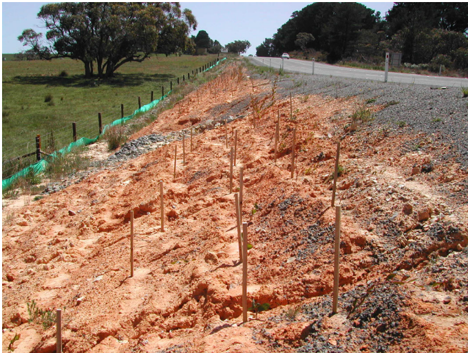
Reactive subsoil, no topsoil, and lack of integrated drainage solution resulted in a batter that had ongoing stability issues.
